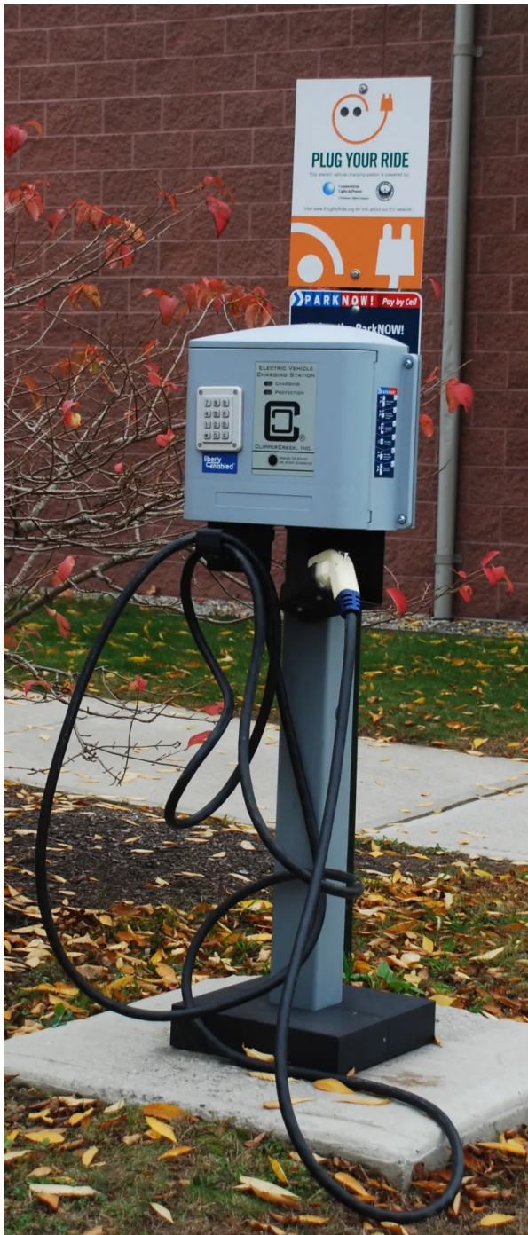
A charging station at the Mansfield Community Center.
